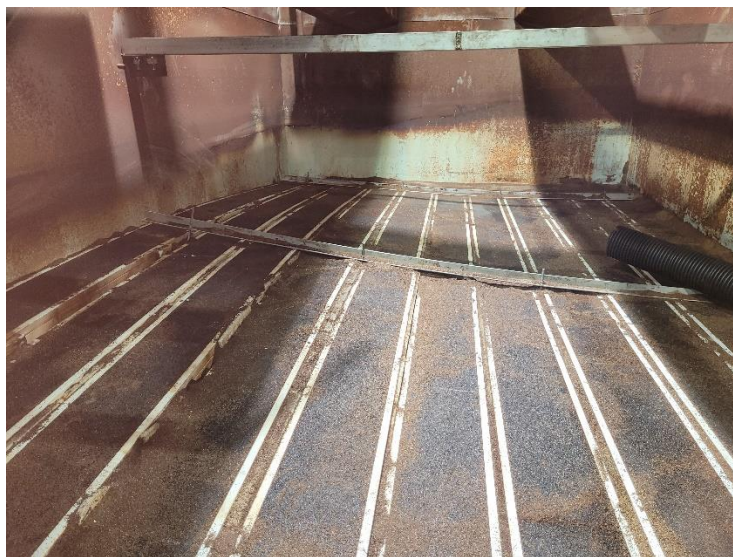
Figure 6-14: Failure of Underdrain Anchors in Filter 2
