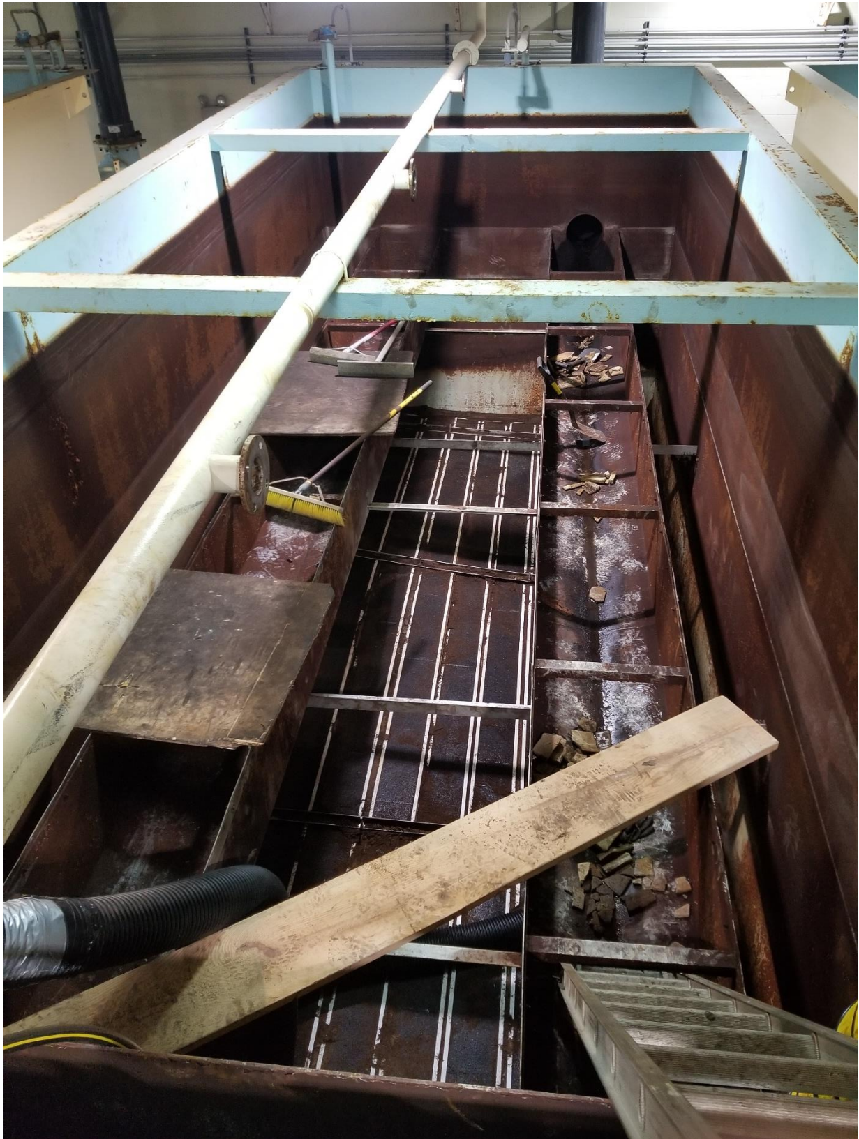
Figure 2. Site photograph showing the interior of Filter #2. The photo was provided by The City of O'Fallon. Pieces of failed grout material can be seen in the photo.
