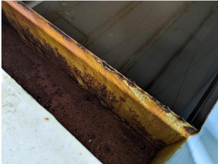
Figure 6-11: Corrosion at Filter 3 Overflow Weir
