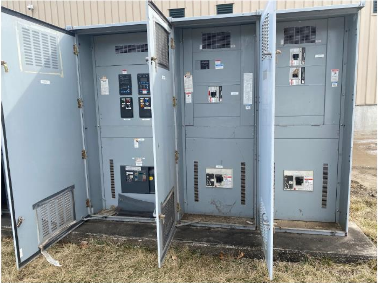
Picture B3: Switchgear 3
