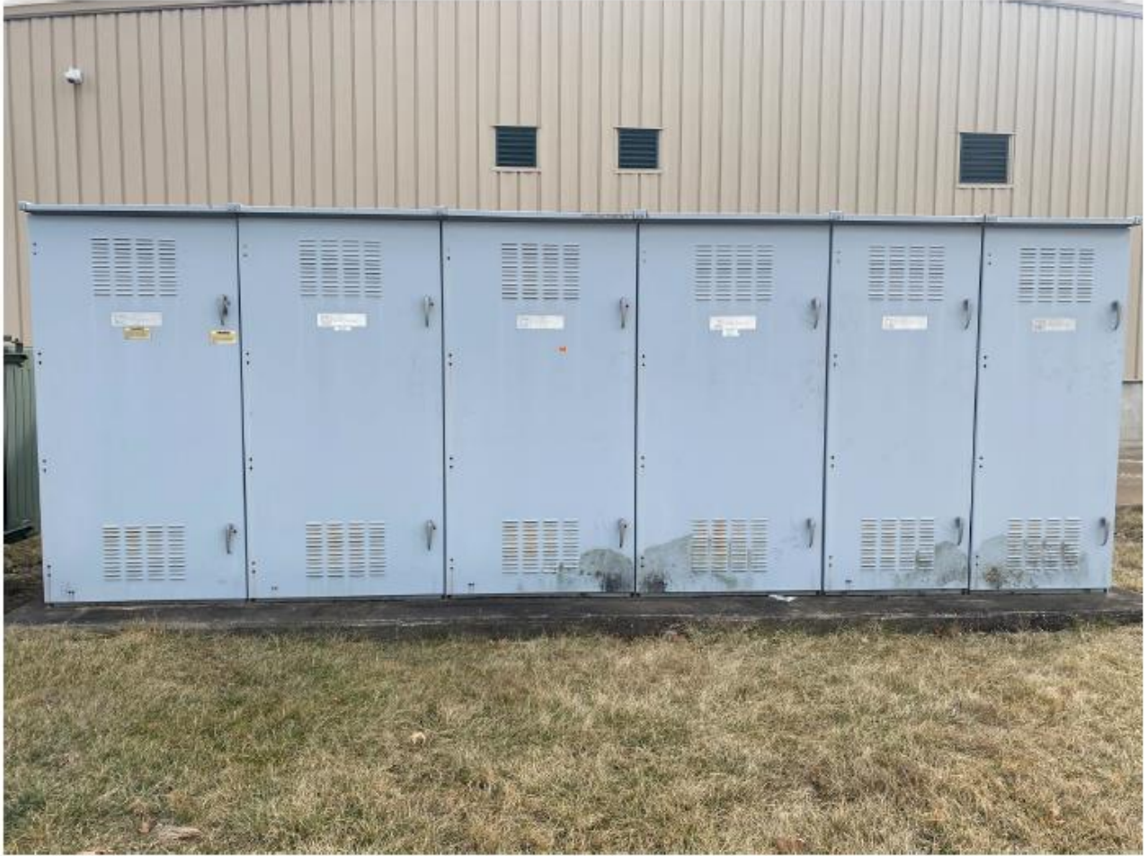
Picture B1: Switchgear 1
