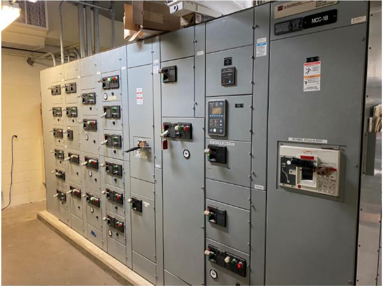
Picture C2: MCC-1B
