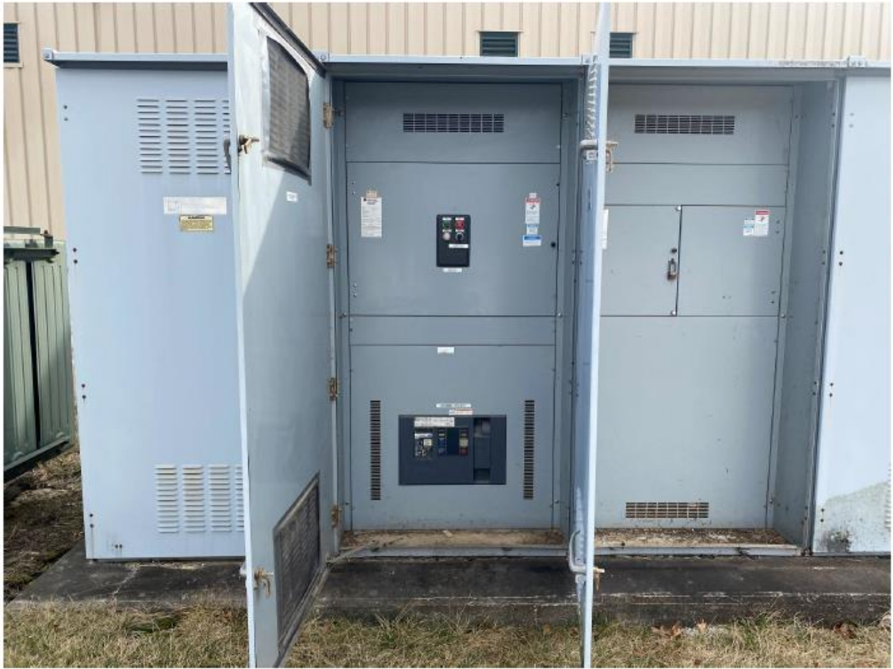
Picture B2: Switchgear 2
